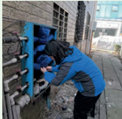
Hanchuan Xinhe Water Supply Co., Ltd. Water Meter Freeze Protection
